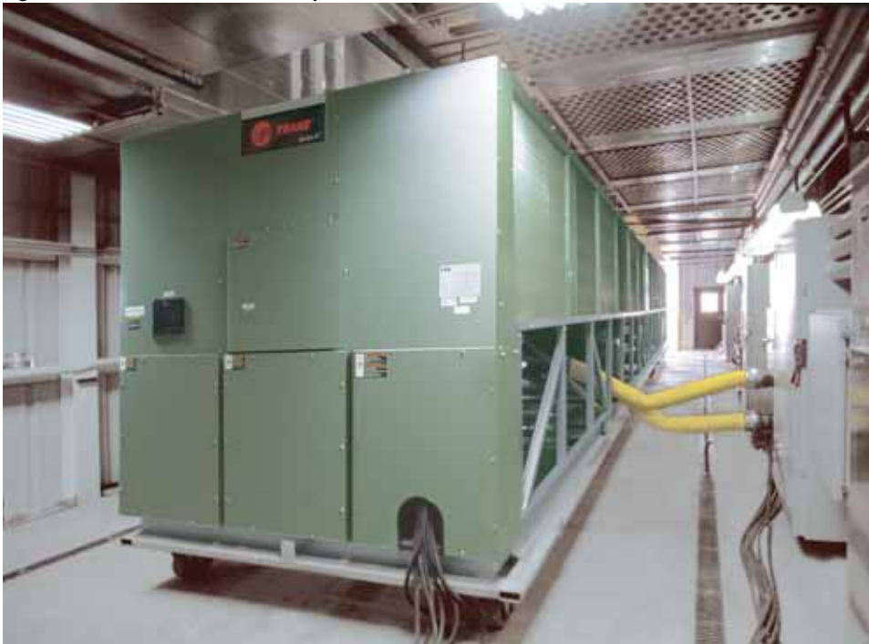
Figure 4. Air-cooled Run Test Facility shown with an RTAC 500 ton unit
