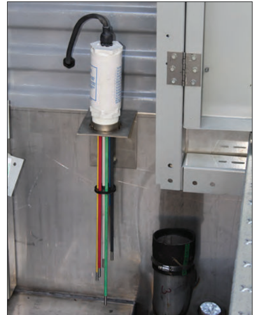
Electric Water Level Control
