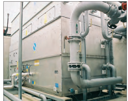
Intake and Discharge Sound Attenuation
