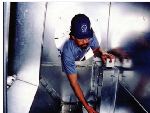
Mechanical Water Level Control Inspection
